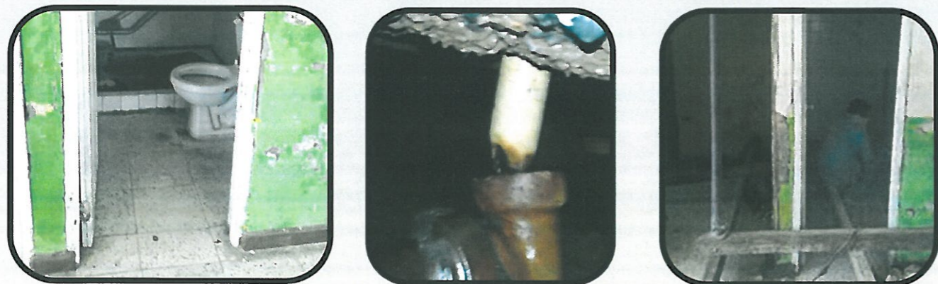
Extremely poor and unsafe conditions inside the safe house
