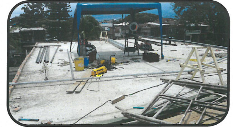
Building work on the roof and below right, Anna, the house mother
